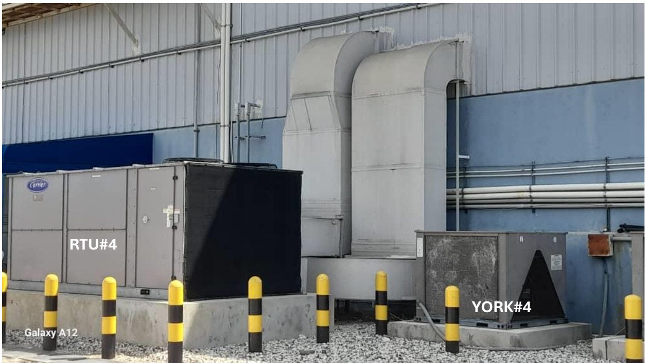
YORK#4 and RTU#4 P4
