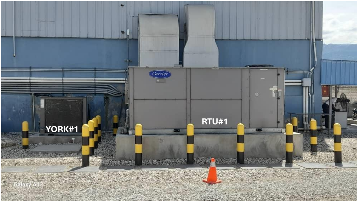
RTU#1 and YORK#1 P2
