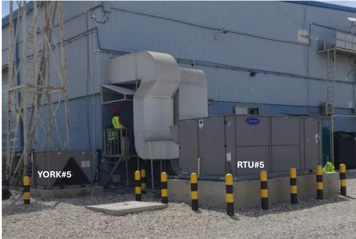
RTU#5 and YORK#5 P5
