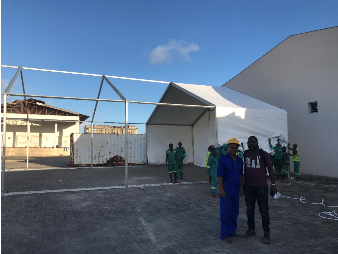
Installation of the first Rubb Hall tent for the emergency warehouse for medicines. Photo: Jan de Jong
