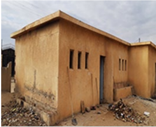
Alwahda school prior to WASH rehab
