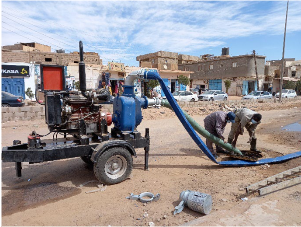
A sanitation company team drains a flooded road in Sabha's Almahdiah neighborhood. PHOTO: LTI 3/Chemonics
